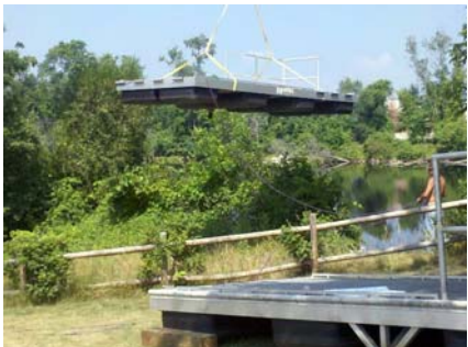
Dock pieces being lifted over the shoreline for gentle placement into the river
